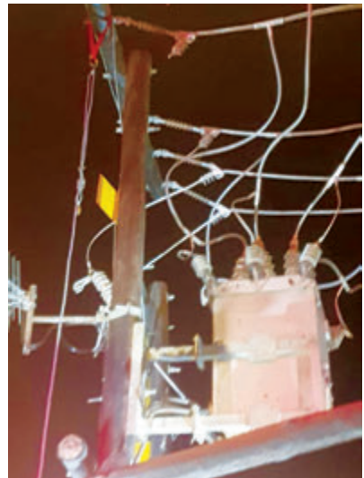
The charred remains of a man were found in-between the Eskom pole and transformer. It took emergency personnel about two hours to remove his body.
